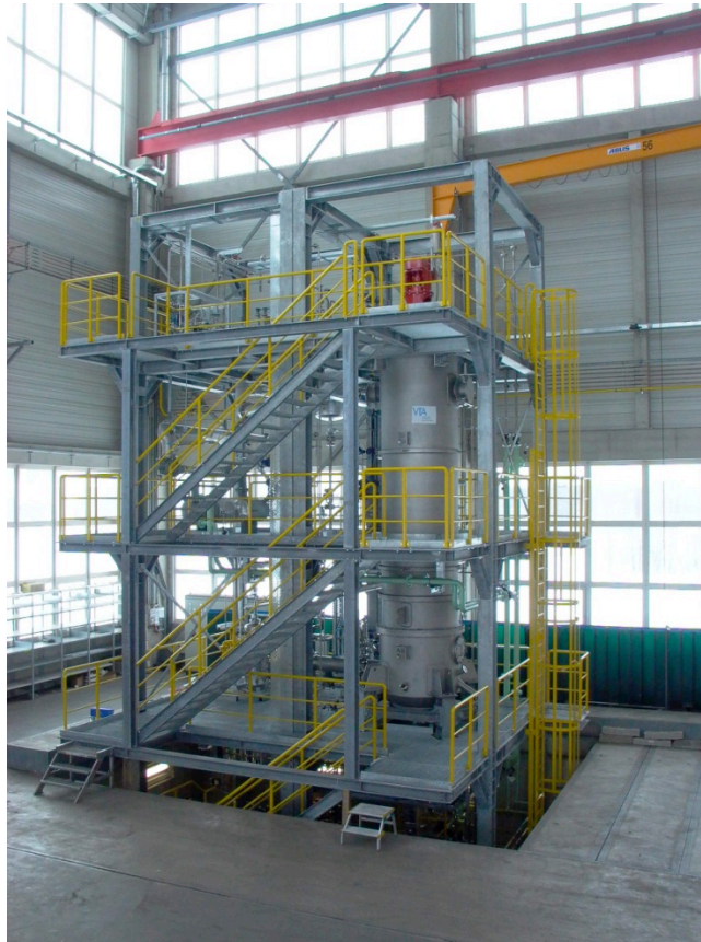
MDI removal plant, skid mounted at VTA workshop after FAT
